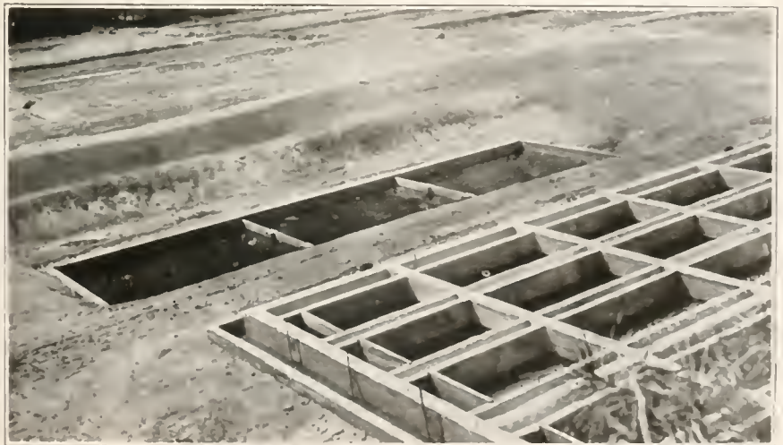
Sewage treatment plant in Yosemite National Park showing Imhoff settling tank in foreground, three sections of sludge beds and ten acres of natural filter beds.
